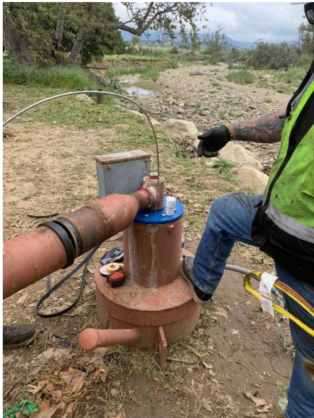
Photo 3. Wellhead landed on well casing. Note new well head with capped 1.25-inch PVC sounding tube on right side.
